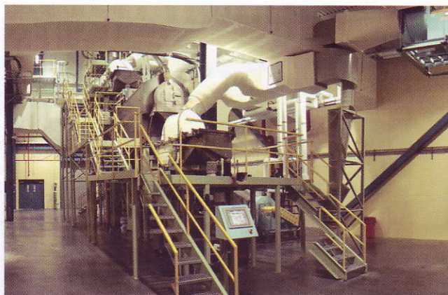
New Compound Equipment
